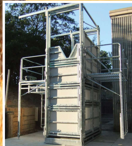
FIGURE 3 Catwalk on both sides of the TAMER™
